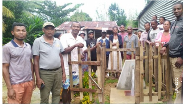
One of the 24 standpipes built to provide access to drinking water for the population of the village of Mandena.
